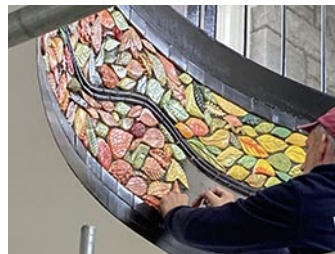
The wall surface was sealed, the black border and "backbone" tiles applied and then the coloured tiles were mortared in. Image Credit: Mary Helen Garsch
