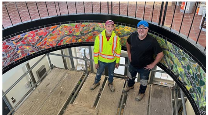
Tile installation and grouting was completed by Gary and Pete from Eastern Ontario Terrazzo & Tile Company. Image Credit: Nancy Martin
