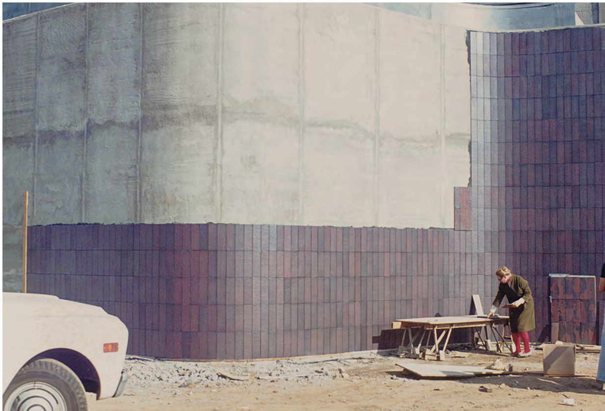
Edith Heath on-site at the Pasadena Art Museum observing the installation of her tile, 1969. Heath Collection, EDA, UCB.
